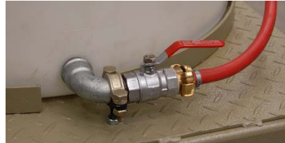
Figure 7b-Water connection at the tank
